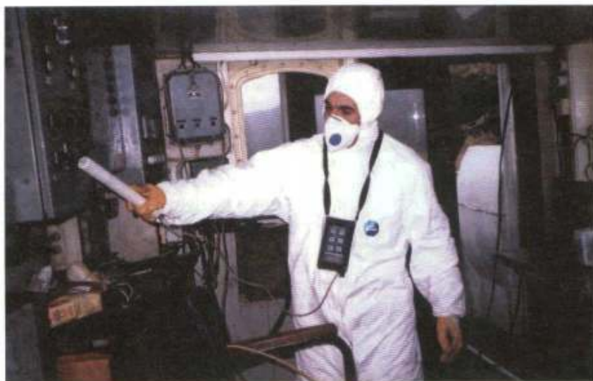
Gas free and radiation checks are integral parts of the pre-demolition assessment of the vessel
